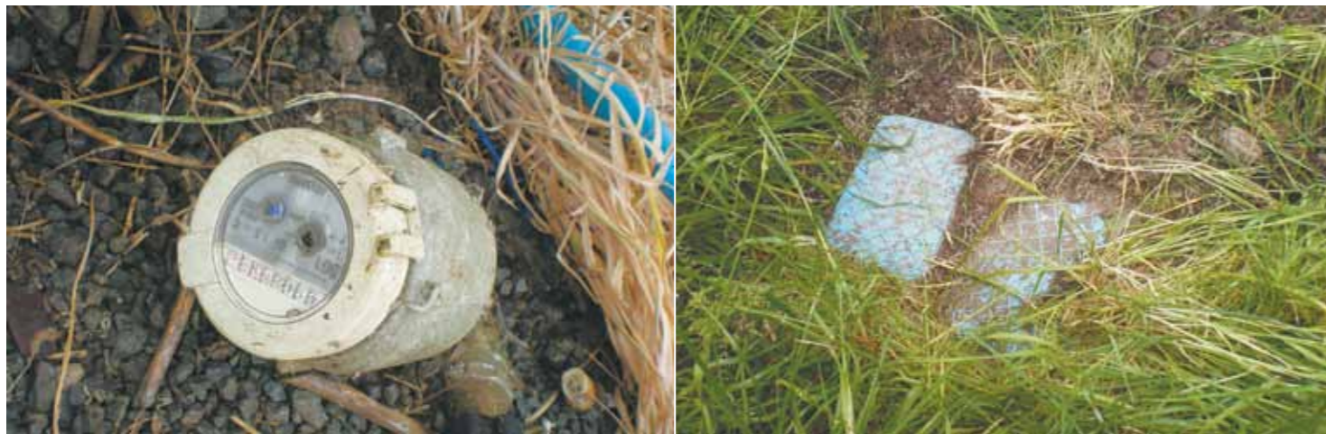
Some examples of installed water meters.
